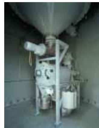
Cyclone screener in a silo skirt
