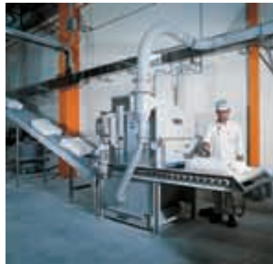
Feeding station with bag cleaning
