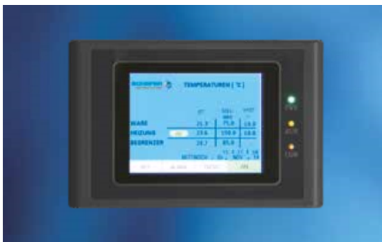
Operator friendly touch panel for heater control
