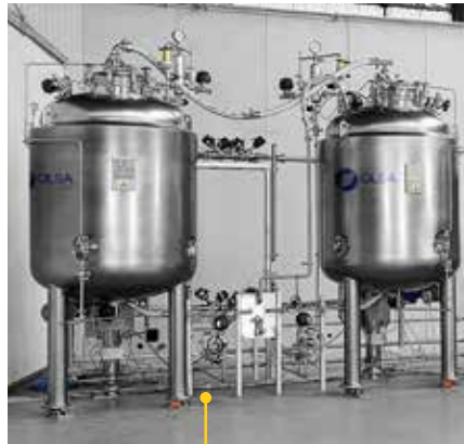
Twin set of preparation vessels with Transfer Panel.
