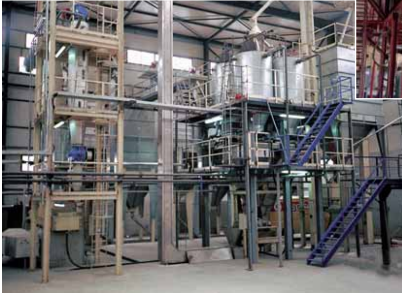
Continuous Parboiling Plants in Greece (Large and small capacity)
