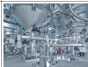
POWDER HANDLING SYSTEM
